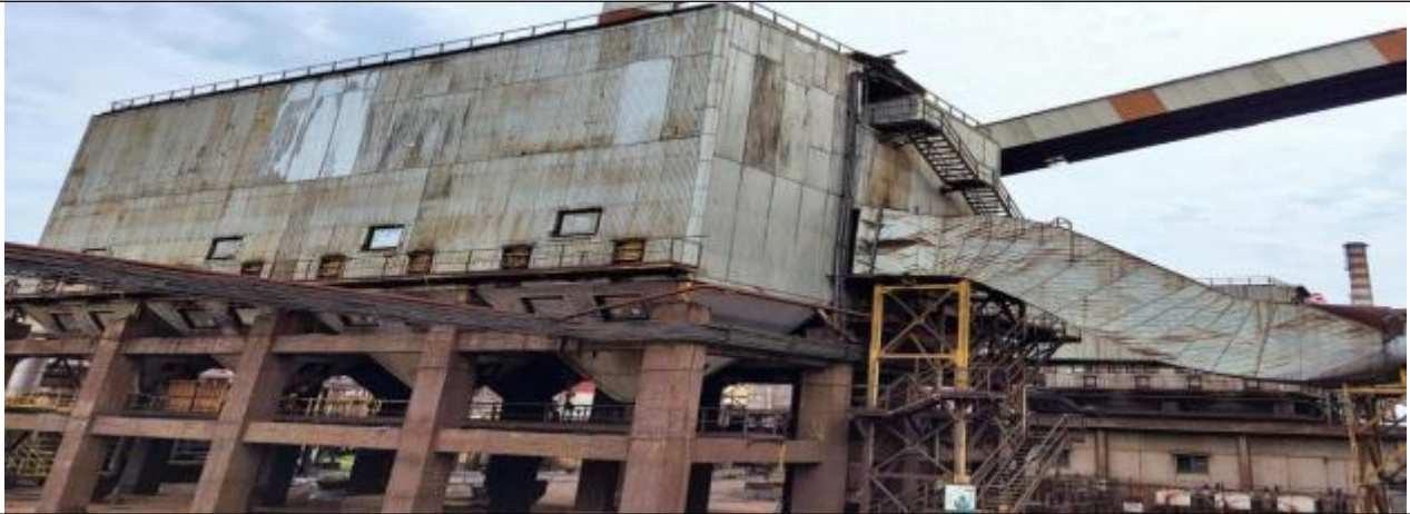
Dry Bottom Ash Handling System-1*80 MW Captive Power Plant
