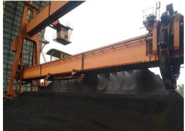
Inbuilt water sprinkler system for stacker at coal handling plant
