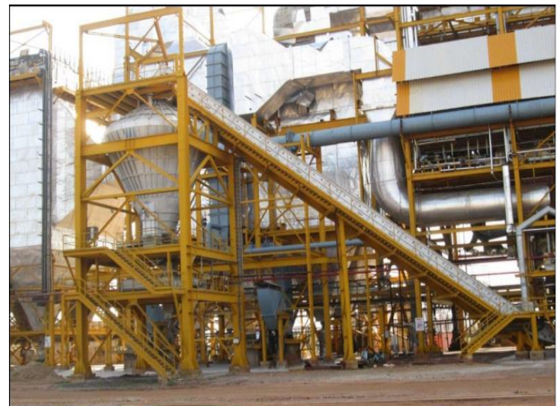
Dry bottom ash handling system-1*80 mw captive power plant
