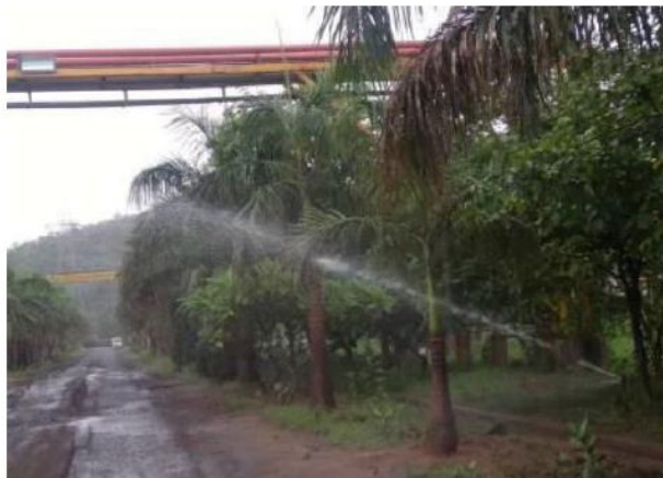
Water sprinkling system for Haulage Road and Green Belt
