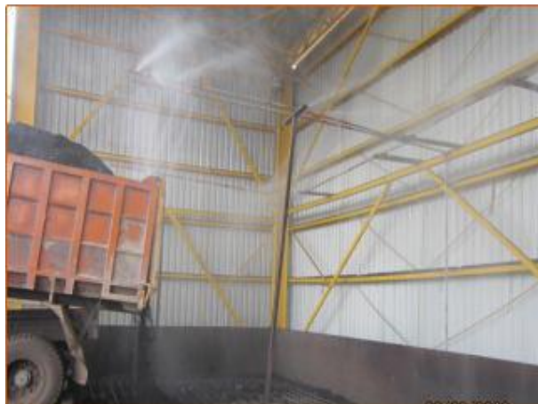
High Pressure Water Sprinkling System
