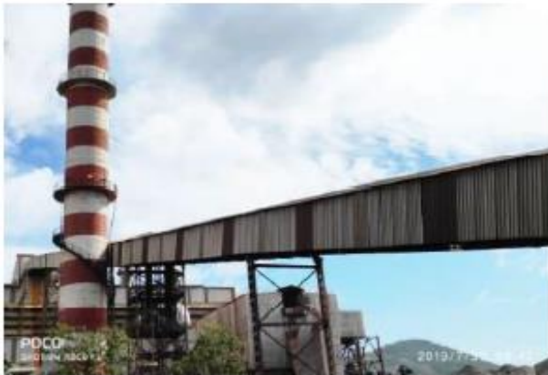
Covered Conveyor Belt at Raw Material
