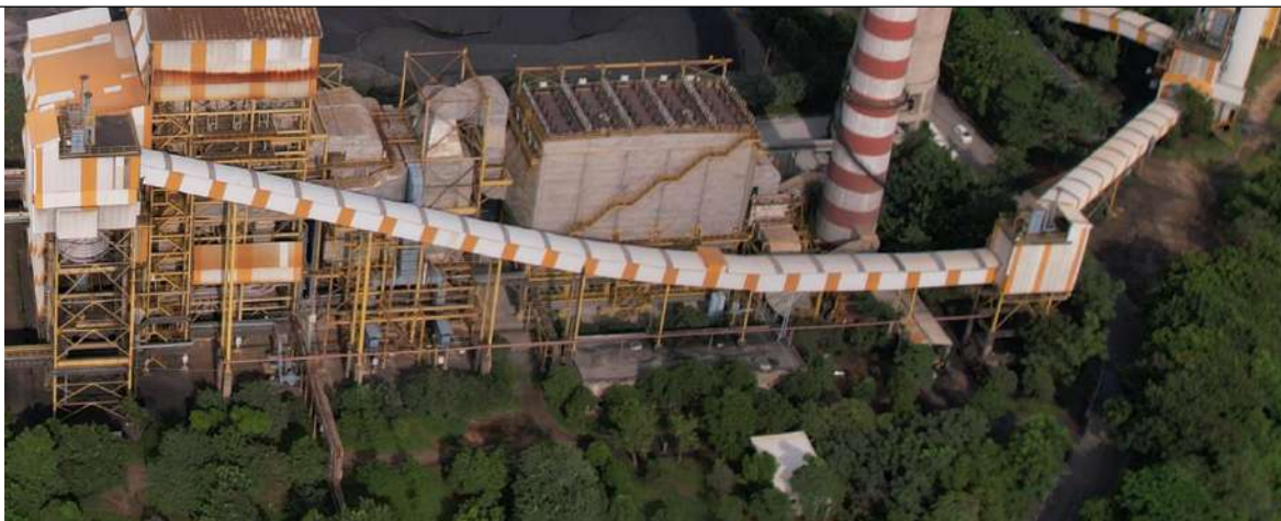
Fume extraction system at furnace
